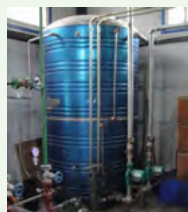
Uninsulated hot water tank
