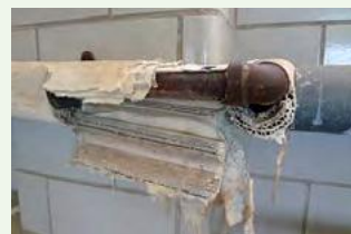
Worn out insulation
