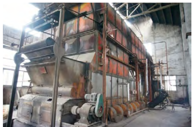
Coal steam boiler
