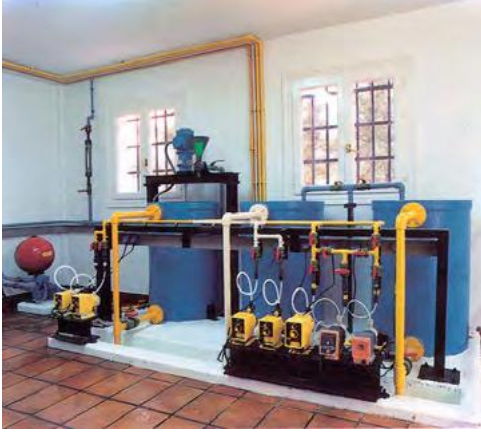
Reagents preparation and dosing system
