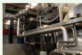
Insulation of process dyeing equipment
