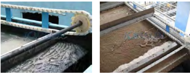
Detail of skimmers removing the floating sludge
