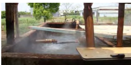
Heat recovery tank
