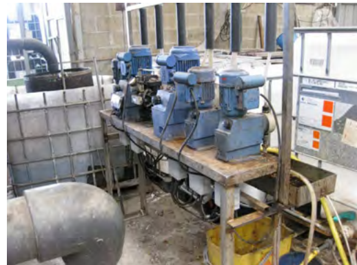
pH regulation addition system on a physico-chemical treatment ETP (Arteixo - Spain)
