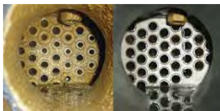
Tubes before & after cleaning Source: universal chemicals.co.in
