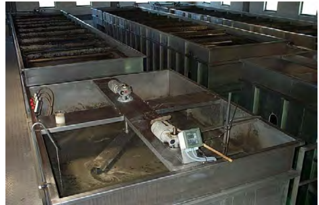
Physico-chemical process based on coagulation-flocculation + DAF Source: WWTP Cee - Coruña
