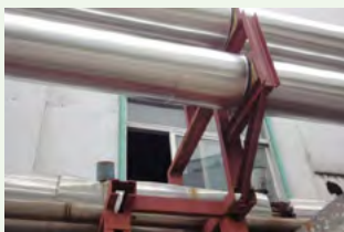
Well insulated pipework
