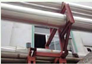
Well insulated pipework
