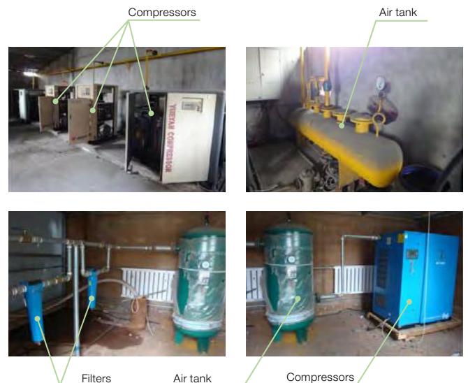
Air compressor, tank and filters in audited mills
