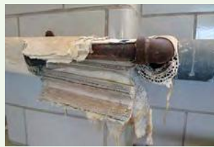
Worn out insulation
