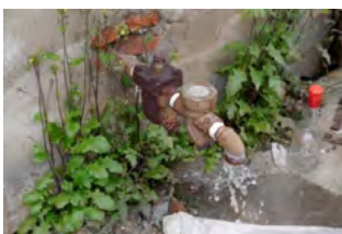
Steam traps discharging on the floor
