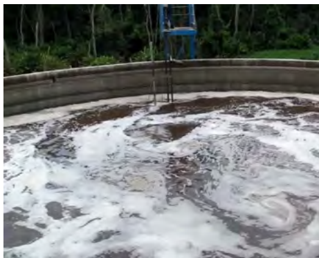
Image of a regulation-homogenization tank
