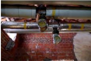
Steam flow meters
