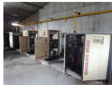
Four air compressors provide compressed air to the system
