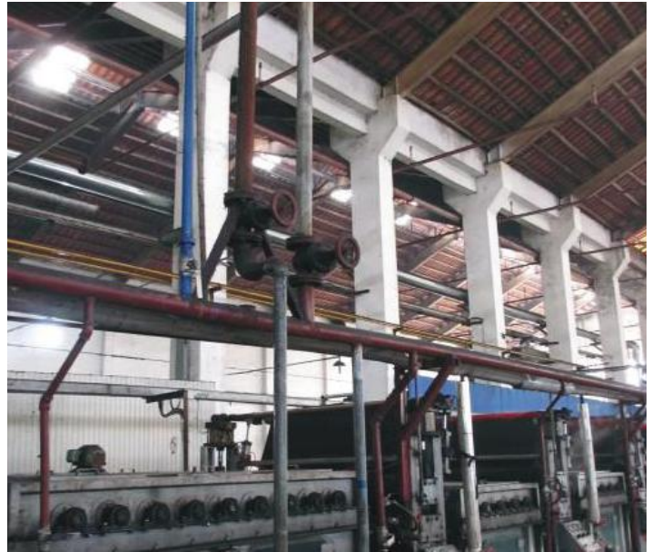
Installed water meters
