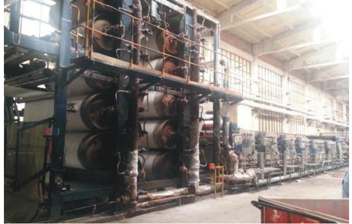
Updated steam trap system for drying cylinders
