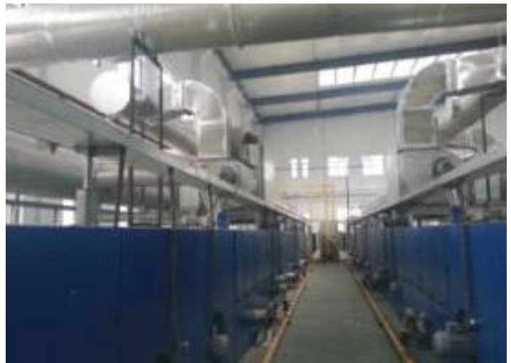
High efficiency heat recovery system on setting machines
