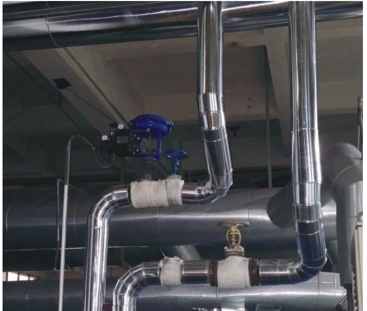
Metering and control system
