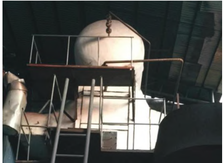
Insulation on Waste Heat Boiler
