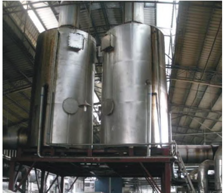
Heat recovery from setting machine exhaust gas
