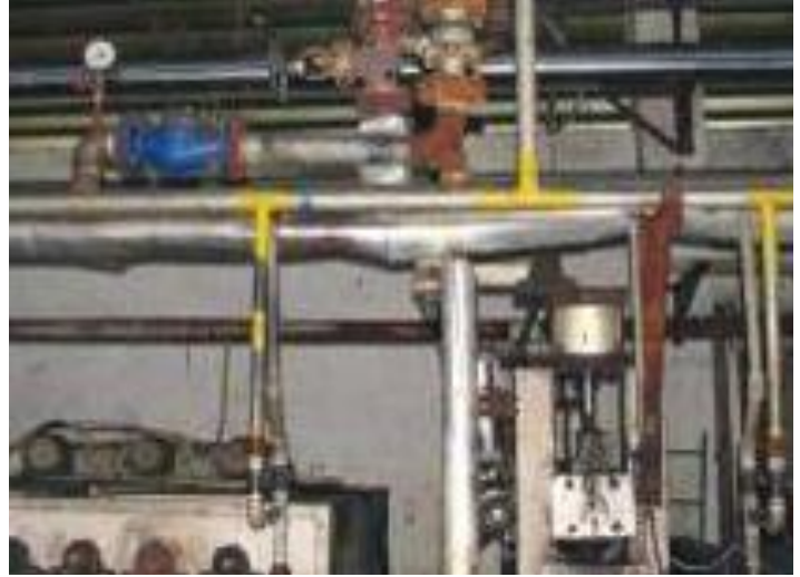
Cooling water recovery pipes system
