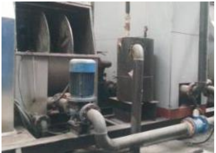
Hot water discharge under high pressure and heat recovery system
