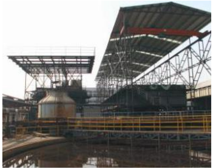
Centralized waste water treatment and reuse system
