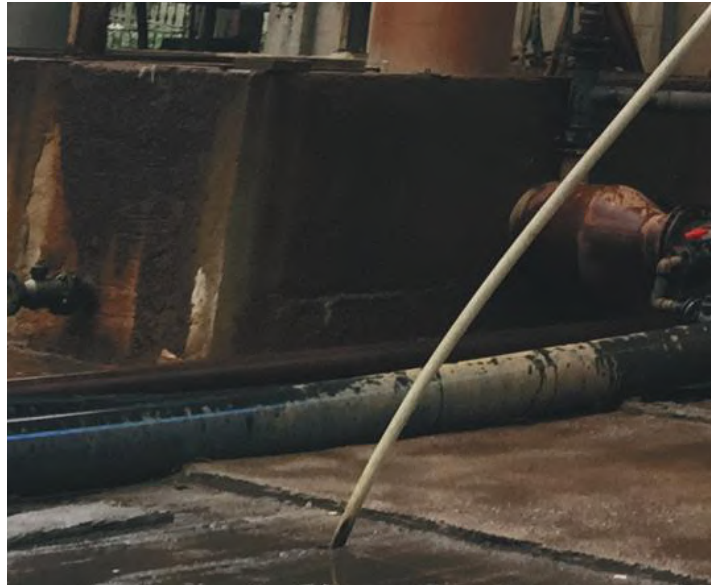
Process water reuse system
