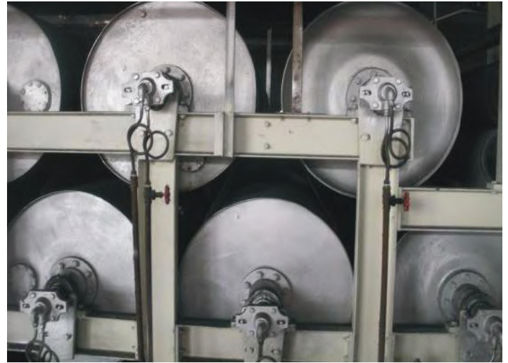
Drying cylinders with insulation on side face
