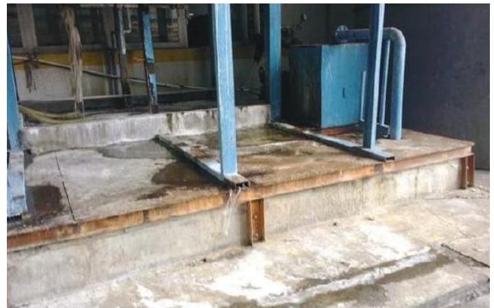
Holding tank for condensate recovery
