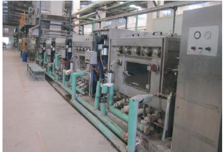
Counter current rinsing retrofit
