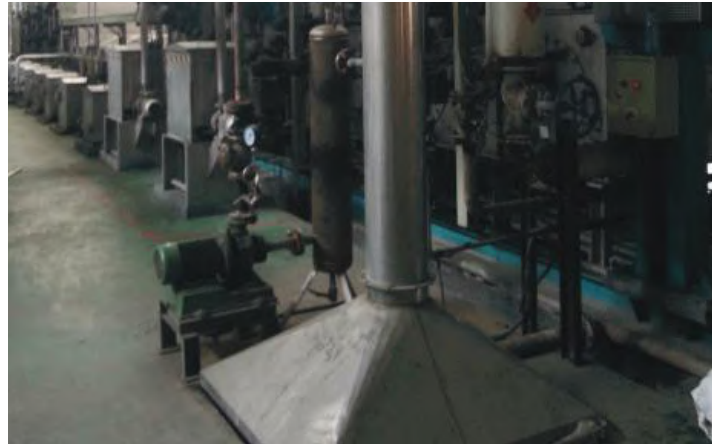
Condensate water recovery
