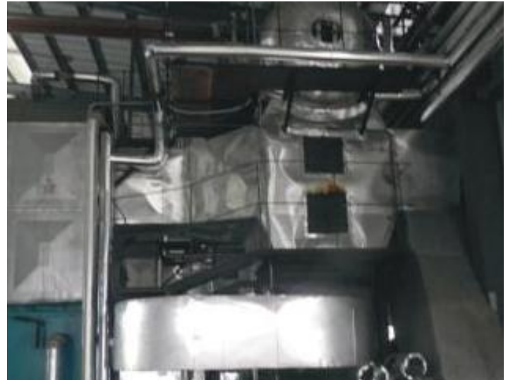
Waste heat boiler
