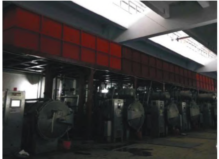
Newly installed cooling water recovery tanks
