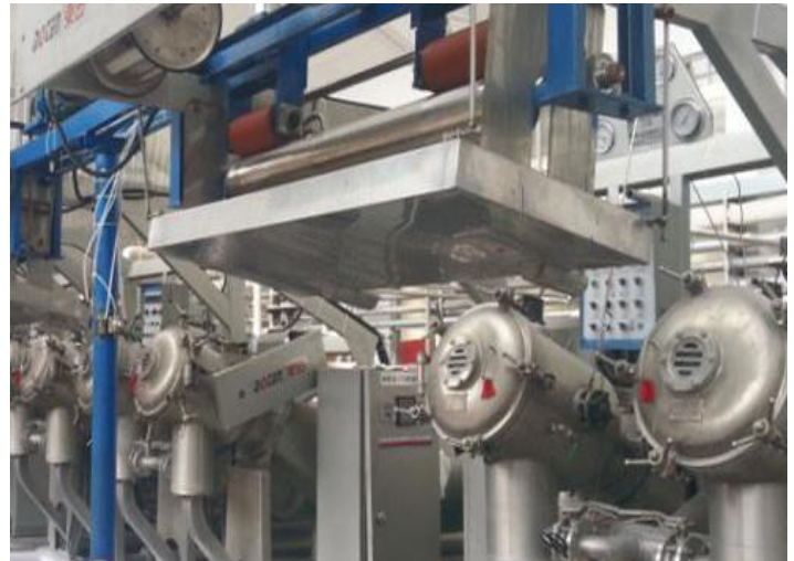
Water squeeze and recovery system
