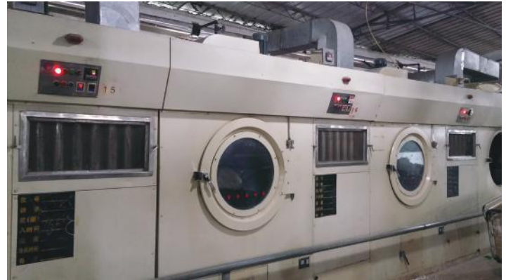
Heat recovery from drying machines
