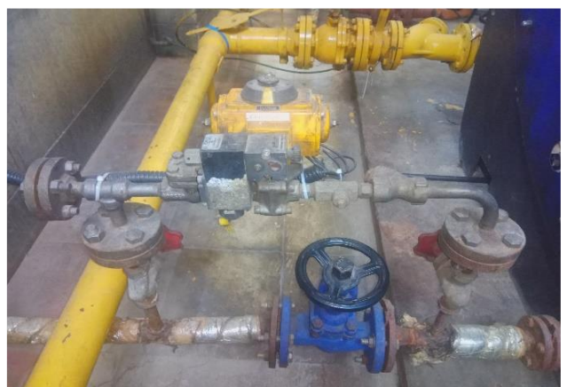
Installed automatic blowdown control system at XYZ
