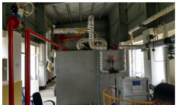
Caustic Recovery Plant (CRP) at Envoy Textiles Limited
