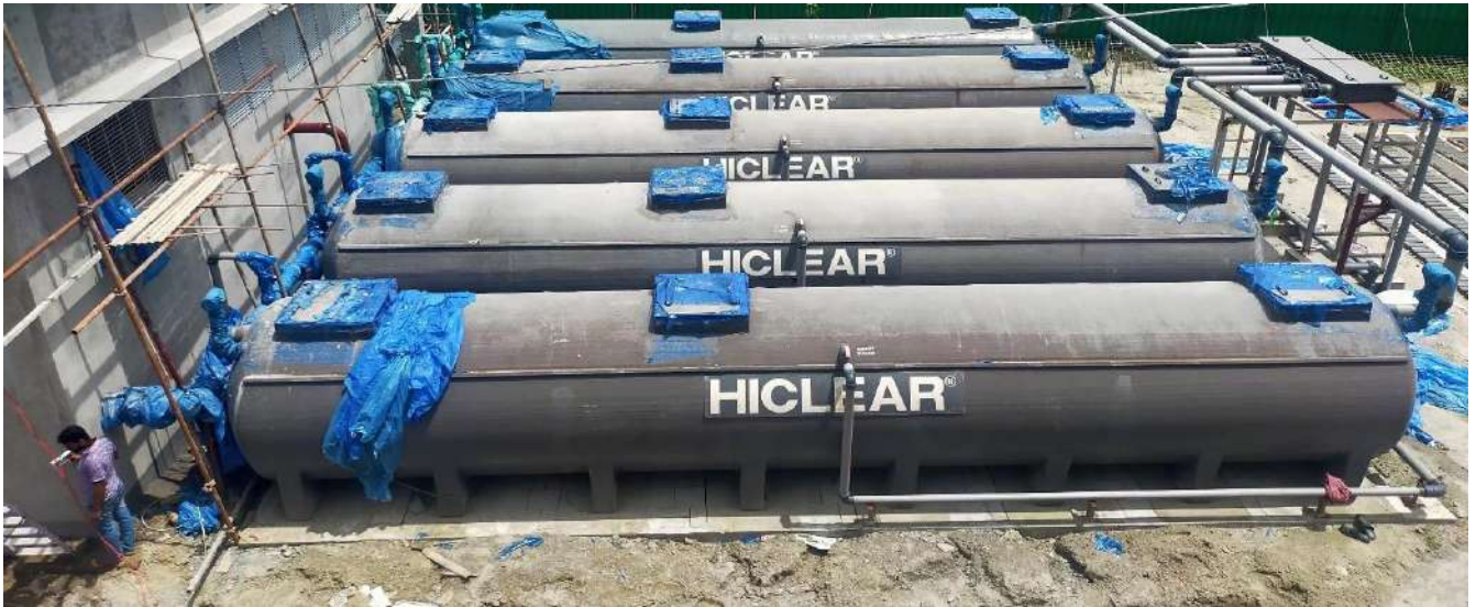
Photo: Sewage Treatment Plant
